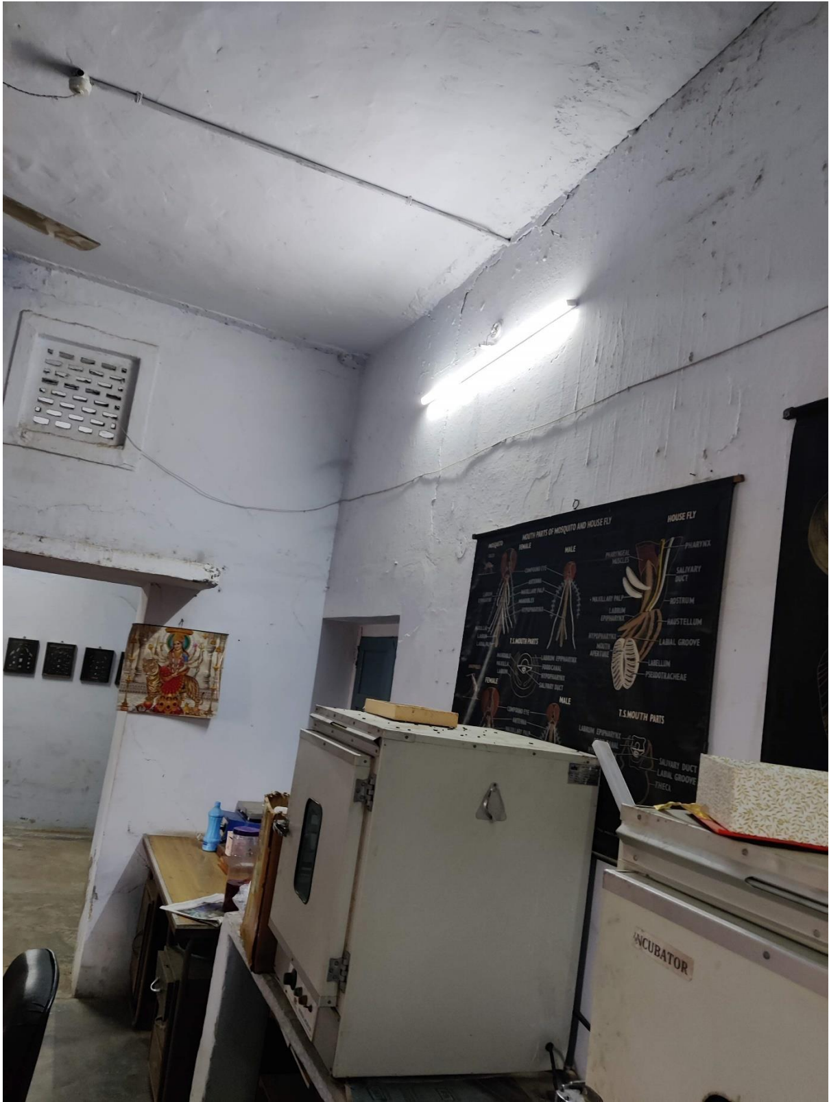
7.1.2 LED LIGHTS IN CLASSROOMS AND LABS
