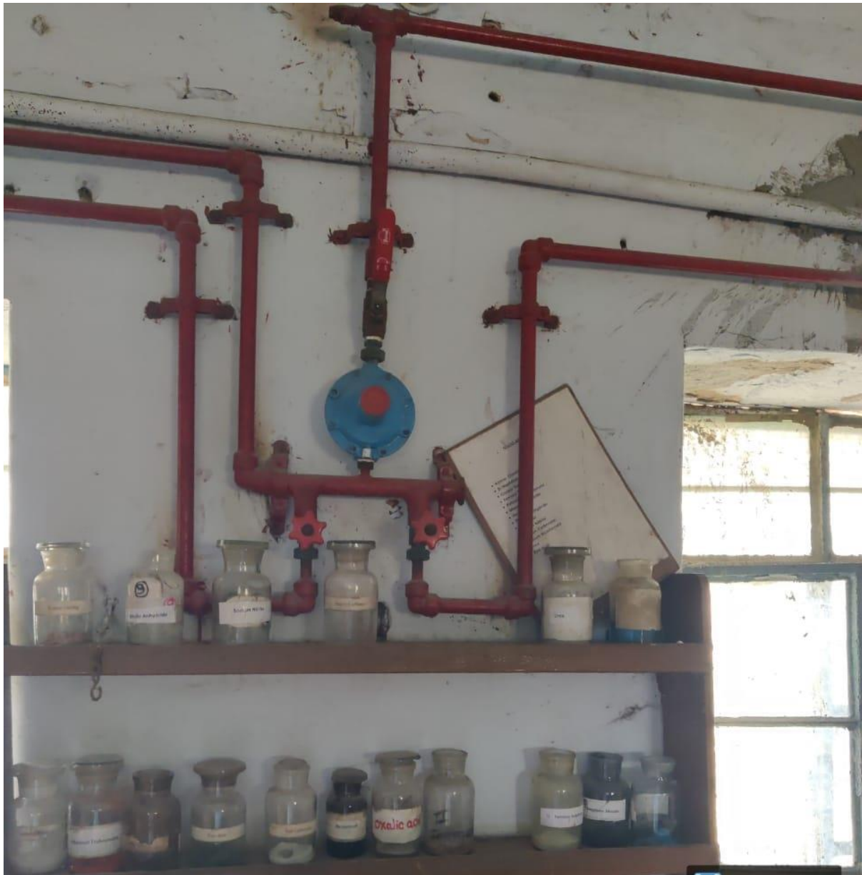
7.1.3 LPG gas Pipeline for burners in Chemistry Labs
