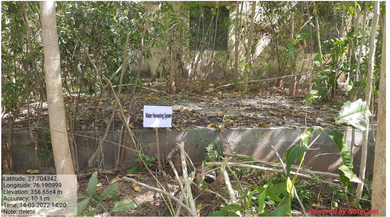
WATER HARVESTING SYSTEM
