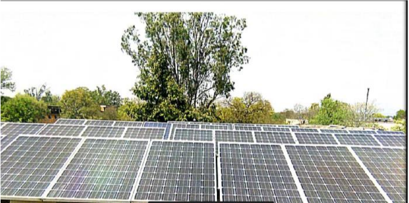
Figure 4- Installed Solar PV of 21k
