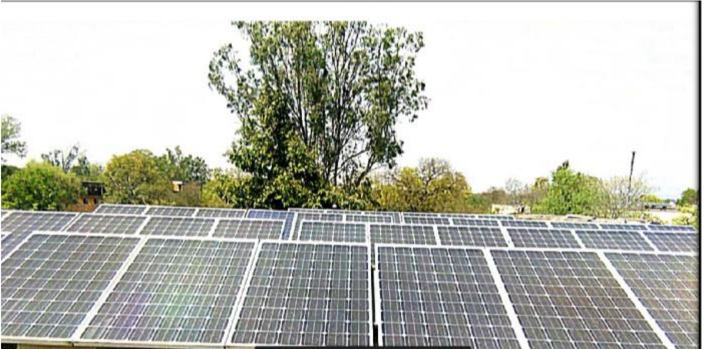
Figure 5- Installed Solar PV of 21kW
